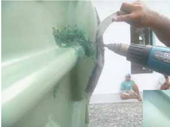
Repairing the top of the tank – using only available plastic – material on the island
