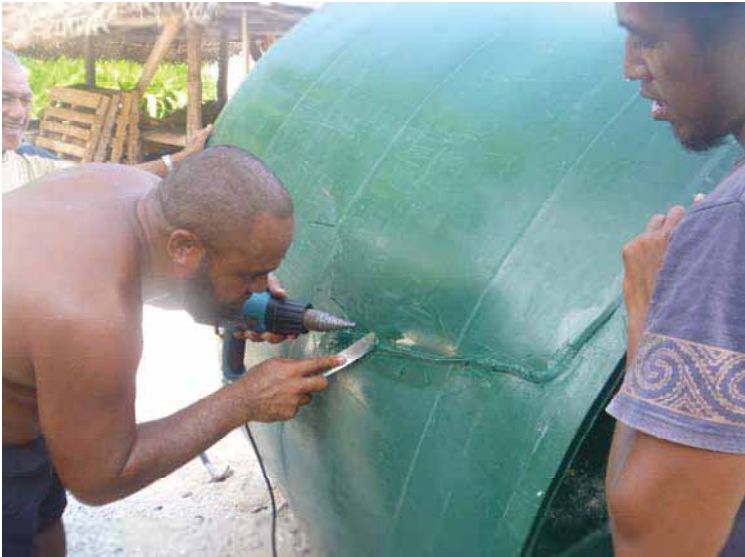
Repairing existing tanks: Using a heat gun to melt plastic sticks onto well-prepared tank surface
